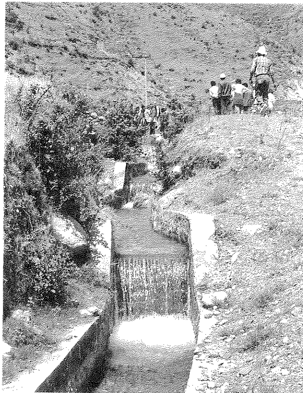
Photograph 51 Eroded Concrete Floor and Masonry Walls of a Vertical Drop Structure
