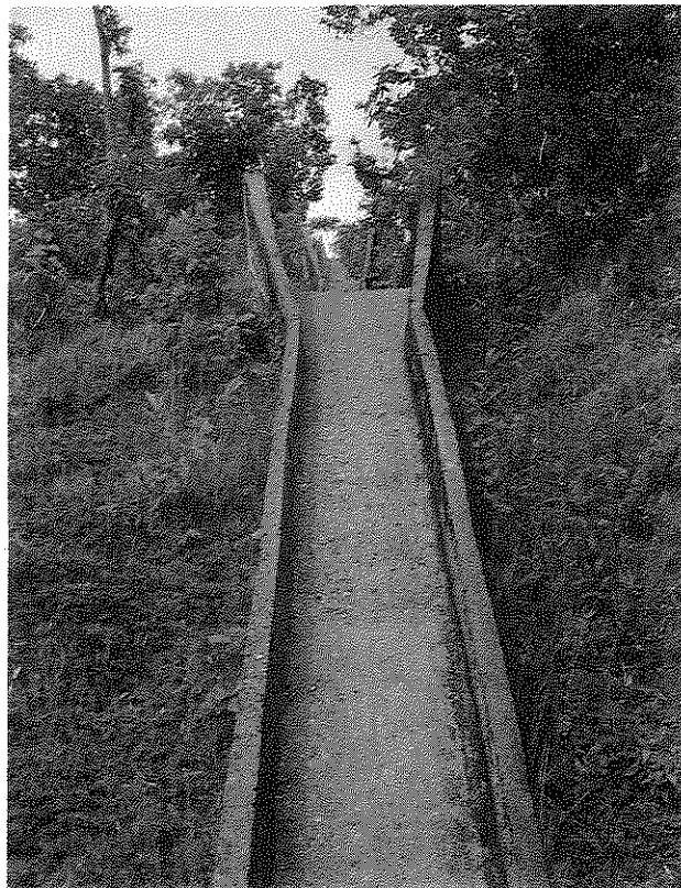
Photograph 5H Eroded Concrete Floor of a Chute Drop Structure
