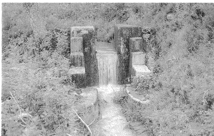
Photograph 5D A Stilling Basin with Insufficient Water Cushioning
