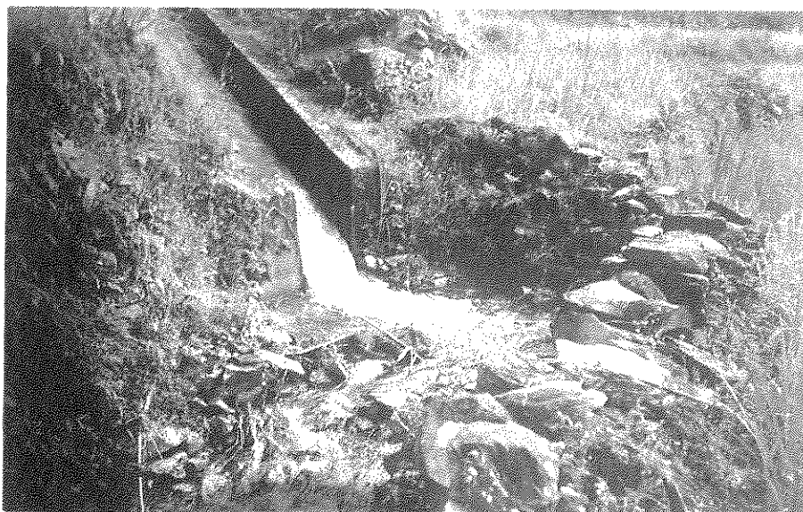
Photograph 5F A Chute Drop Structure with an Inadequate Stilling Basin
