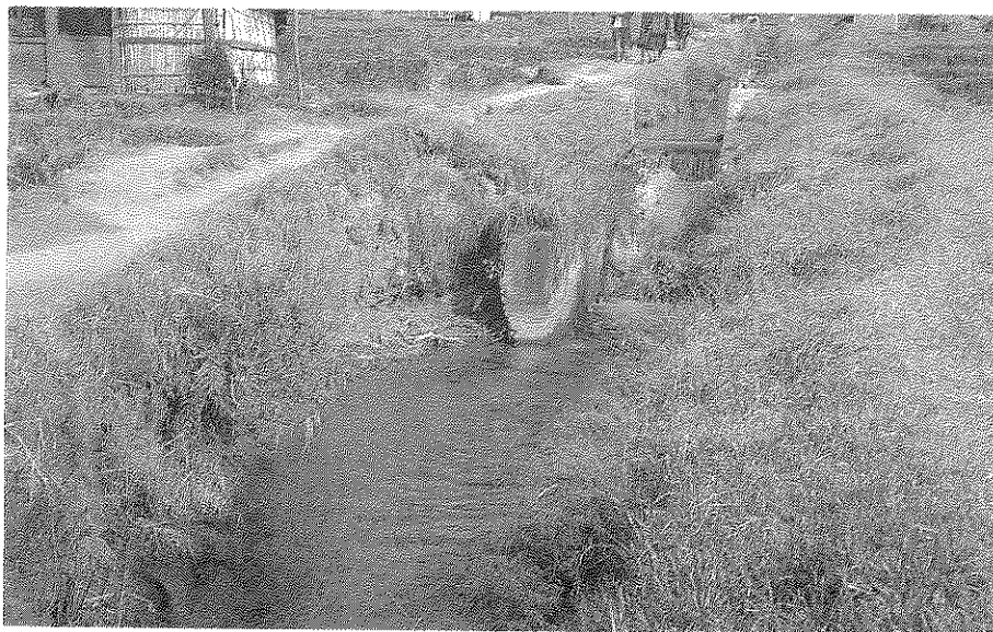
Photograph 5G A Vertical Drop Structure with Inadequate Stilling Basin and Downstream Protection
