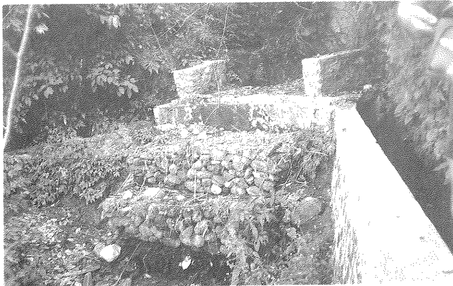
Photograph 4L Eroded Downstream Area Below the Super Passage due to Inadequate Protection
