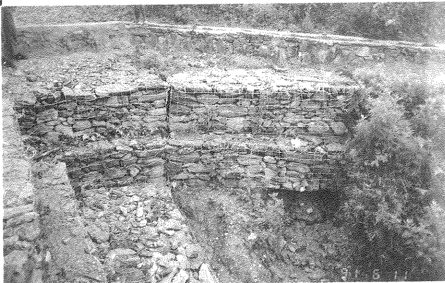
Photograph 4M Eroded Downstream Area Below the Super Passage due to Inadequate Apron
