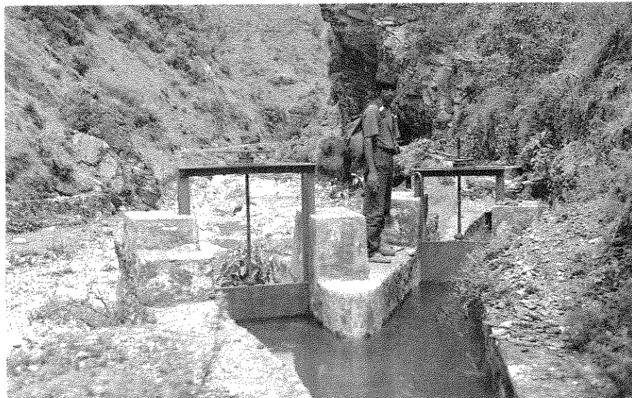
Photograph 2B Settling Basin with a Frontal Flush Gate and a Head Regulator
